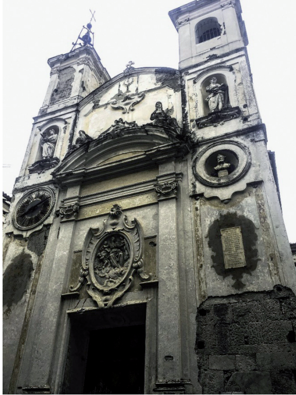
Figure 2. Sessa Aurunca (Caserta), Church of San Giovanni in Piazza. View of the façade on Corso Lucilio, highlighting the mediocre state of conservation of the finishings (photo: Francesco Miraglia).
