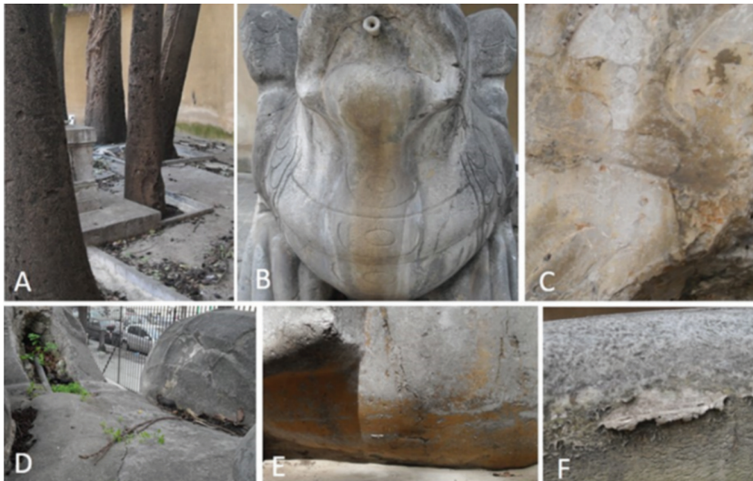
Figure 2. Deterioration signs. (A) Trees behind the fountain; (B) front of dragon with evidence of water leaching, rusty patina; (C) other patinas and dirt on dragon's wing; (D) vegetal remains on dragon statues or plants inside fissures and loss of materials due to the presence of metal brackets; (E) colored patinas on lower part of dragon; (F) flaking of material composing the rim of fountain.
