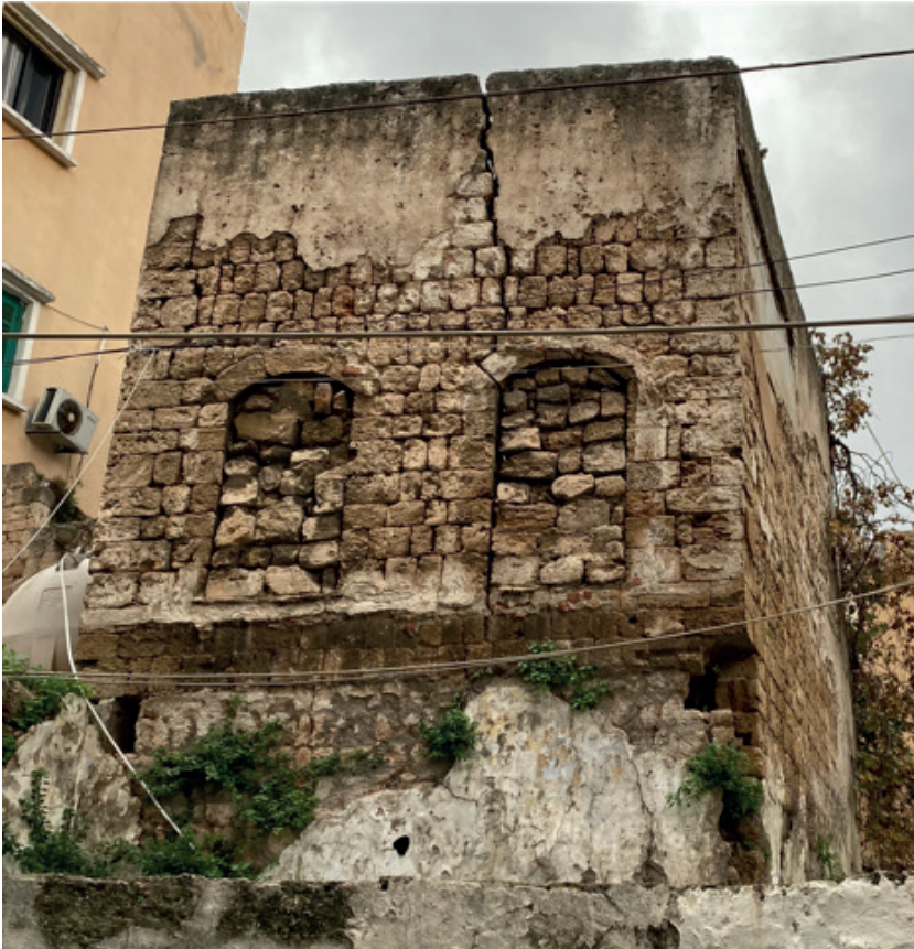
Figure 11. Cracks and plantation on the facades of Dr. Yaacoub Labban habitat building (Source: Authors, 2023).
