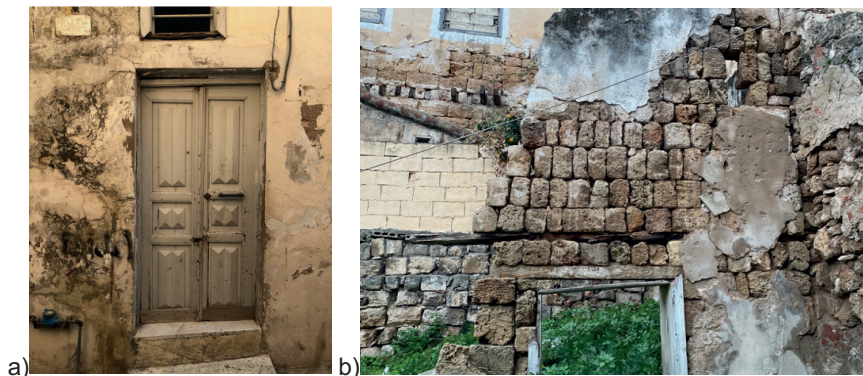
Figure 6. Building 318/12. a) Door façade; b) and ruined building walls (Source: Authors, 2025).
