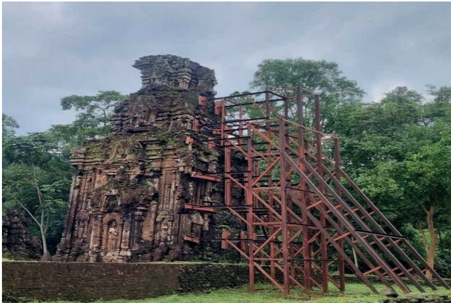
Figure 1. View of the entire B3 tower tilting and settling more than 3 degrees toward the southwest, as captured in this photo by Dr. Dinh Van Trong.
