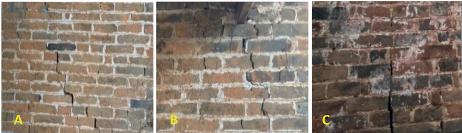
Figure 4. Images of the cracks in the horse-head wall of the wind-rain bridge. (A) Crack area 1; (B) crack area 2; (C) crack area 3.
