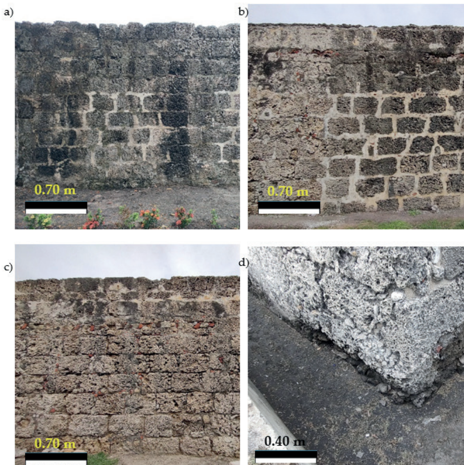
Figure 2. An example of deterioration on the city walls of Cartagena de Indias. a) and b) widespread rising damp on the walls; c) widespread deterioration of mortar; d) rising damp at the cornerstone of the Santo Domingo Bastion.
