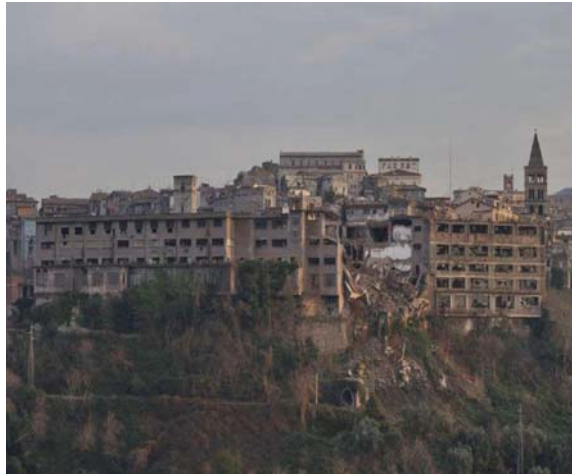
Figure 4. Present day situation (2020): result of the massive collapse of 2009 on a section of road, "Via degli Stabilimenti", that runs through a tunnel (Source: Municipality of Tivoli).
