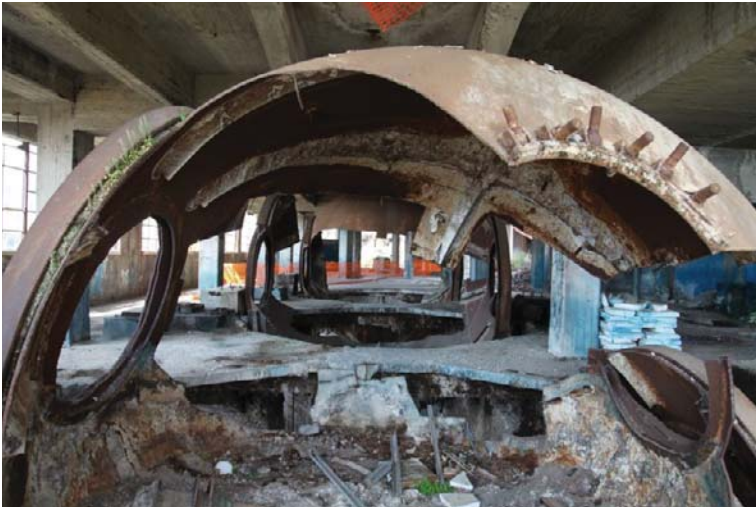
Figure 7. Image taken at elevation of the boilers area (204 meters a.s.l.) (Source: Carlo Vannini).
