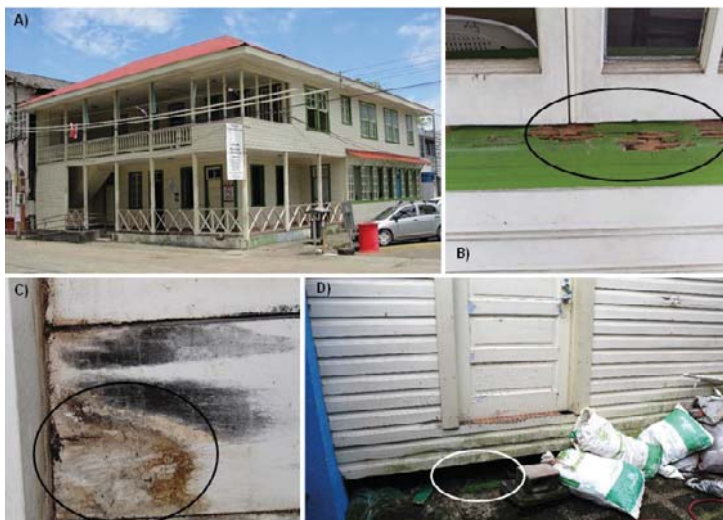
Figure 4. Antigua Capitanía de Puerto (AAA - Type 1 - 01). A) South and East view of the façade; B) Damage caused by insects (termites) (indicated with a black circle); C) Damage caused by humidity and fungi (indicated with a black circle). D) Presence of vegetation under the structure (indicated with a white circle).
