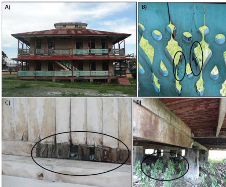
Figure 3. Casa Misionera de la Iglesia Bautista (W - Type 1 - 01). A) Front view. B) Damage caused by insects (termites) (indicated with black circles). C) Damage caused by humidity and fungi (indicated with a black circle). D) Presence of vegetation under the structure (indicated with a black circle).
