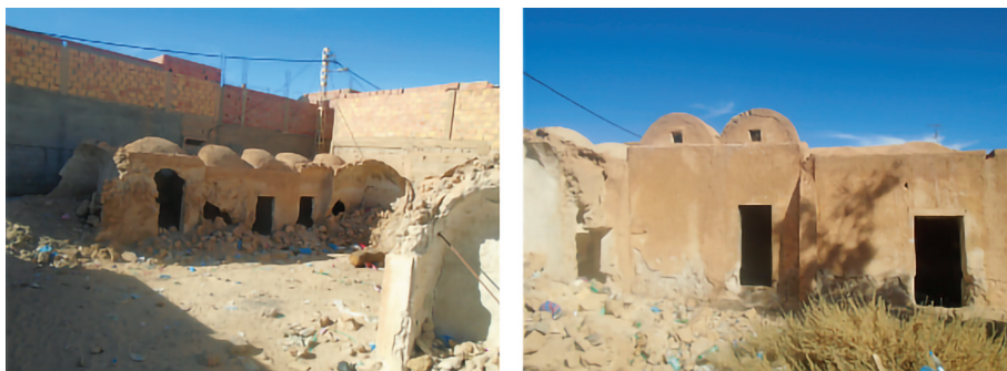
Figure 9. Views of demolished houses in Guemar showing domed and barrel-vaulted units (Source: authors, 2022).
