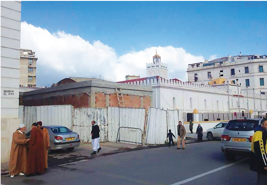
Figure 7. The Djama'a El Kebir Mosque in Algiers –by its status as a listed monument, it is given special protection from any intervention, but here we note that its integrity has been endangered by an illicit construction.
