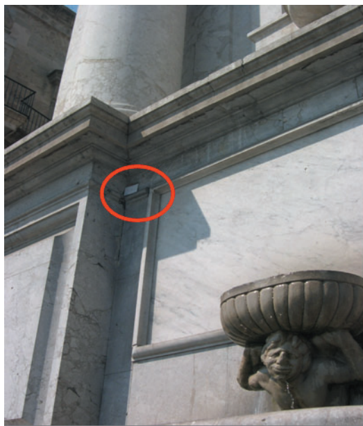
Figure 16. Location of corrosion coupon on Porta Felice (side Foro Umberto I).
